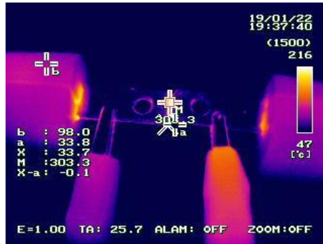
Figure 4.16: Large amount of heat generated at the base of the blade could be the result of the heat transmission from the brass metal.
